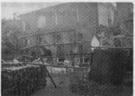
Figure 7 A seven storied building after collapse
