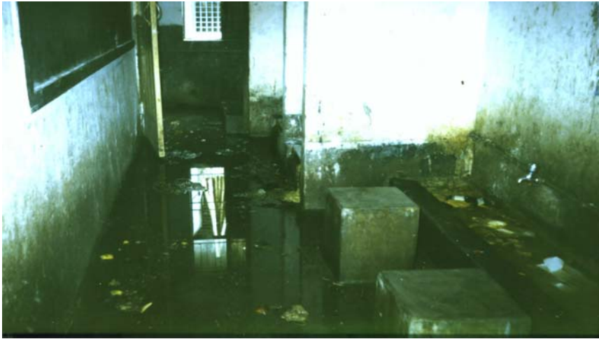
Figure 8: Poorly maintained, unhygienic toilets
