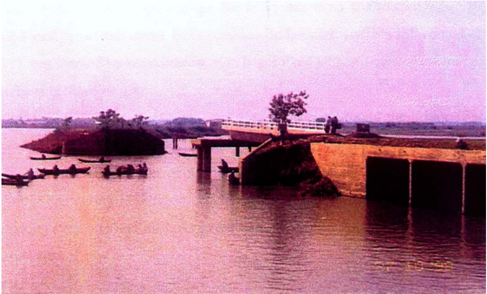
Figure 6: Washed away Turag-Bhakartha bridge on Turag-Bhakartha road near Amin Bazar close to Dhaka-Aricha road at Savar during the 1998 flood (Date: 27-10-98)
