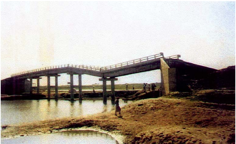
Figure 5: Settlement of Pier-1 of Turag-Bhakurta bridge on Turag-Bhakurta road near Amin Bazar close to Dhaka-Aricha road during the 1995 flood (Date: 25-02-95)
