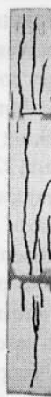
Fig. 6 : Mode of failure and crack pattern columns with precast ferrocement jackets divided into three segments
