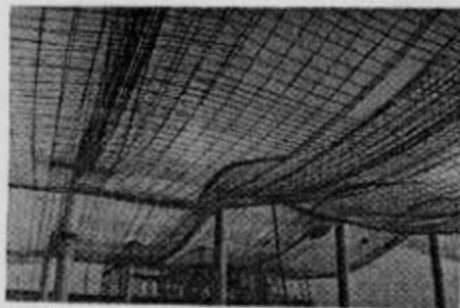
Fig. 3 Reinforcement of roof slab as well as inverted beams being held by cracked columns after the collapse of under construction roof slab in the adjoining areas
