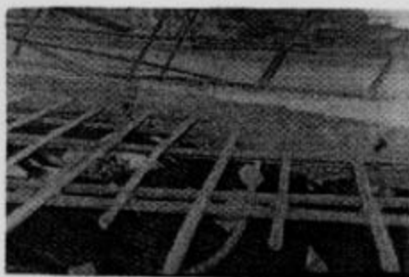
Fig. 5 Part of the collapsed roof slab showing closely spaced top and bottom bars in the slab
