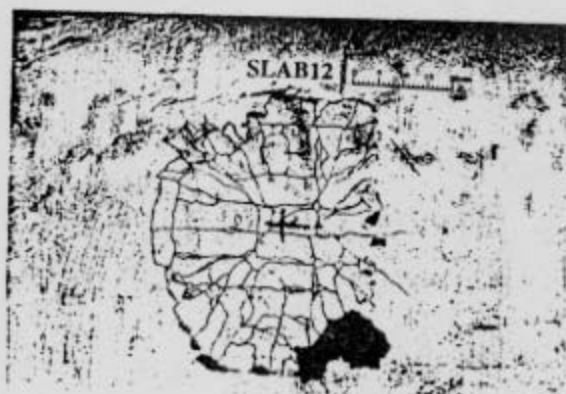
Figure 5: Crack Pattern on Bottom Surface of SLAB1, SLAB3 and SLAB12 Tested
