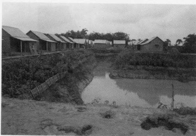
Figure 1 : Steepness of pond, Narrow streets deteriorating by washing away, in rainy season, The unsettled land causing sinking of plinths Proshika Palli in Diabari, Manikgonj.
