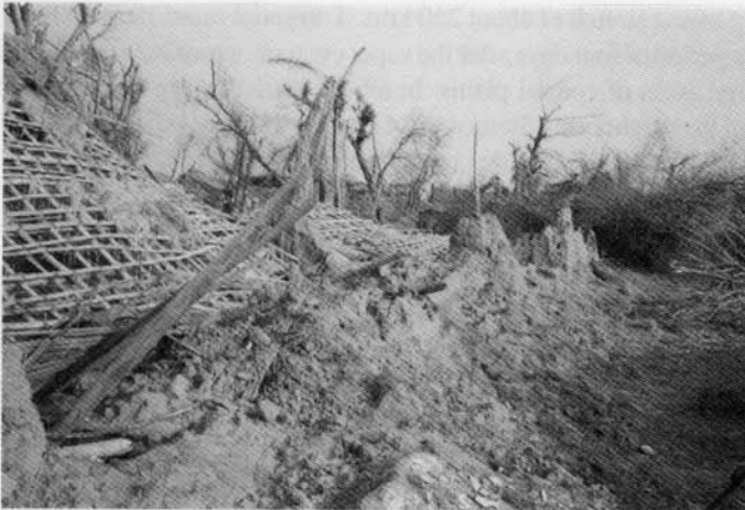
Figure 3 : Performance of houses of mud, thatch and bamboo is quite poor during the cyclone. These houses were damaged very severely during the recent cyclone.
