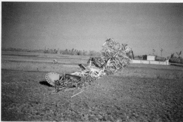
Figure 4 : The traditional modes of communication like radio, television, etc. were hugely damaged due to this cyclone. The transmission tower of the Cuttack radio station fell down on November 29, 2000 disrupting the broadcast of the warning messages
