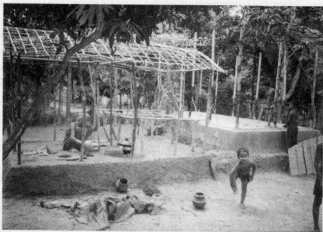
Fig. 5 : The demonstration house after completing the stabilised plinth (on the left: new kitchen being built , later roofed with recycled cement bags
